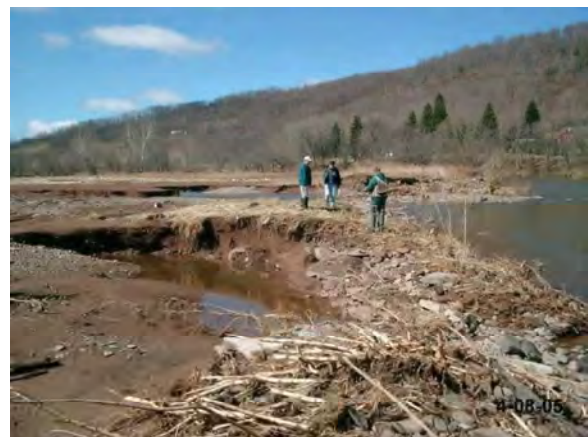
Figure 3.12 Berm that was breached in 2005 storm event
