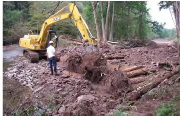
Figure 3.16 Root wads were placed in two layers with large boulders or logs to hold them in place
