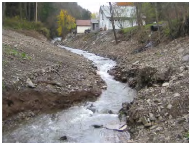
Figure 2.16 Headcut on Third Brook in Walton, NY
